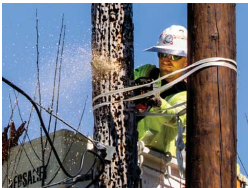
24 - PG&E Wildfire Abatement Team Replacing Damaged Woodpecker Granary Pole - Corral de Tierra, CA - March 2020.jpg
